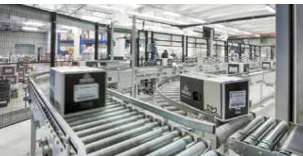
Case/Tote handling conveying systems.
